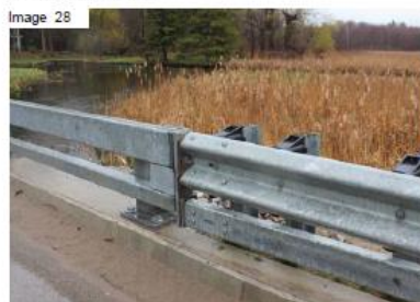
SE guide rail connection
